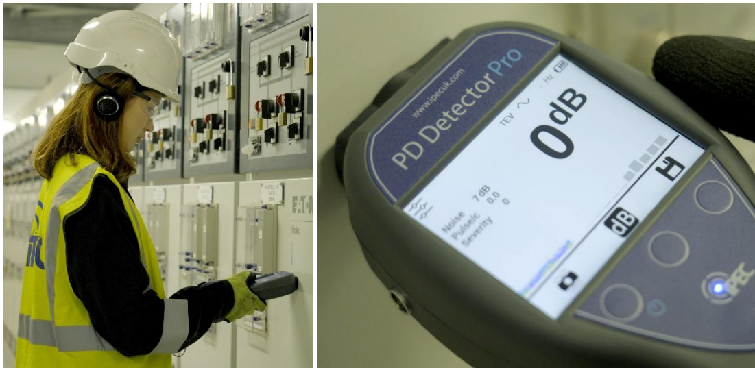
Figure 20 - Photos showing the PD Detector Pro surveying a switchgear panel in TEV mode.
