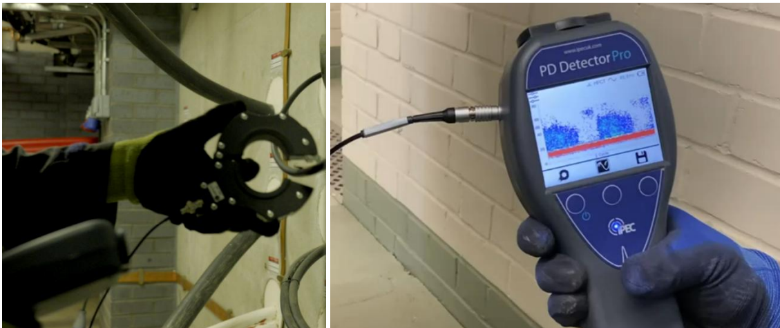
Figure 27 - Photos showing the HFCT sensor being coupled around the cable earth and connected to the PD Detector Pro.
